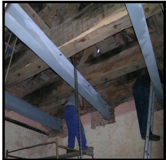
The new RSJ beams supporting the old timber bell frame support beams.
