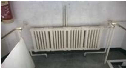
Retain existing iron radiators on the first floor and reutilise them on the ground floor
